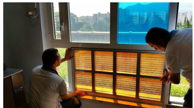
Fig. 7. Photovoltaic generating façade set-up.
