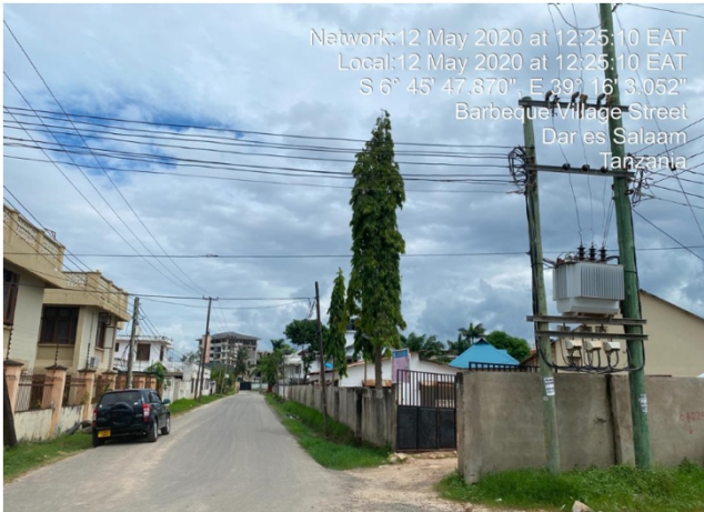
Fig. 1. Study Area SDPN BBQ Village Transformer
